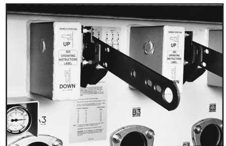
▲ Single phase interrupter operating handles.
