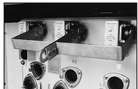
▲ Three phase interrupter operating handle.
