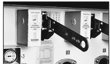
▲ Single phase interrupter operating handles.
